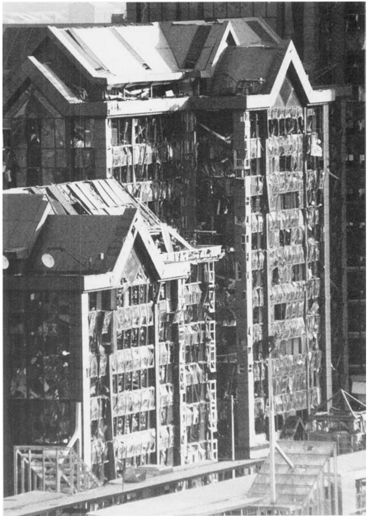
Damage caused by the February 1996 terrorist bomb exploded in London's Docklands
